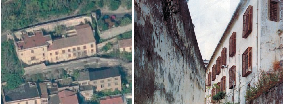
Figure 4. The ex-monastery of San Pietro a Maiella e San Giacomo in Salerno, Italy.
