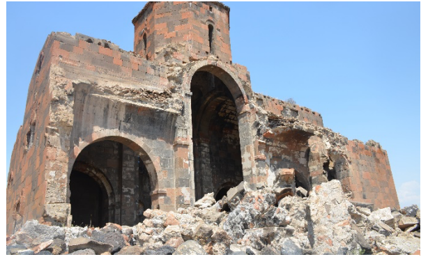
Fig. 7 Collapse and urgent structural threat at Mren, 2022 (Photo: WMF)
