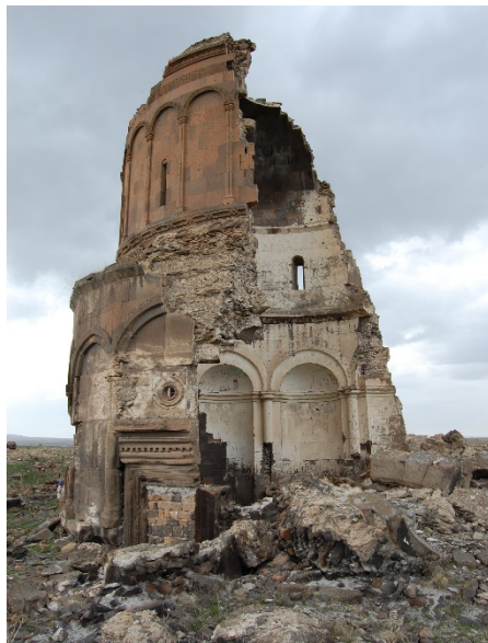
Fig. 4 The Church of the Holy Redeemer in dire condition (before physical intervention), 2009 (Photo: WMF)
