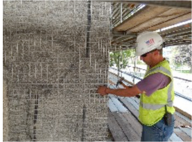
Fig. 3 Unity Temple, Chicago, the shotcrete in the recent restoration works, 2015, Harboe Architects.
