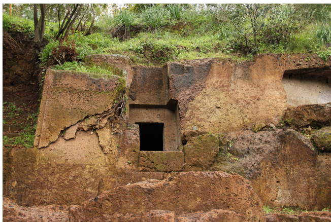
Figg. 19-22 Several situations in which the lignified roots of tree and shrub species have produced severe damage to artefacts
