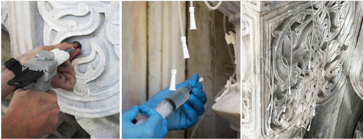
Figure 3. Strengthening and stabilization of column capitals with epoxy resin injection and stainless-steel threaded rods (photo F. Betül Değirmenci Breitenfeldt, 2023).
