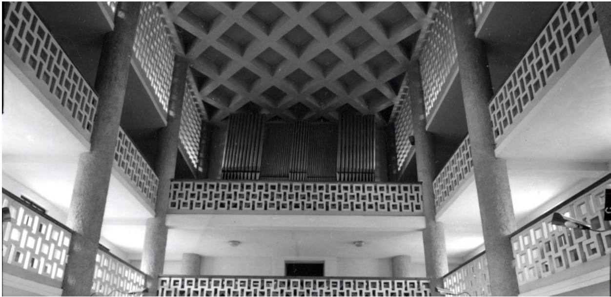
Figure 1. Reinforced concrete ceiling and skeleton with emporas as new solution of the war-destroyed gothic church in Handlová, Slovakia: after the Second World War, the original medieval shape of the church was restored, but its interior already declared the time of its creation, and the defunct vaults were only to be evoked through a new reinforced concrete ceiling. © Archive of The Monuments Board of the Slovak Republic.
