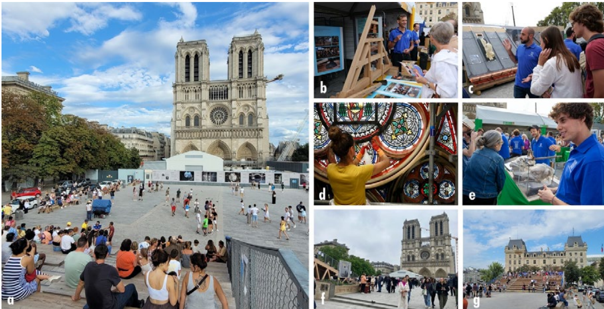
Fig. 3 The Paroisse de Notre-Dame, Paris: the Village du chantier and the wooden public observation staircase on the restoration site (photo A. Komenda 2022 (b, c, d, e) and A.R.D. Accardi 2023 (a, f, g)).
