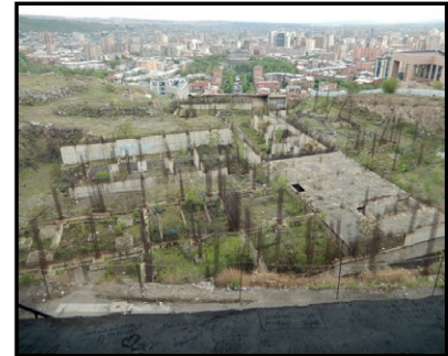
Top ruined areas over the complex staircase and under the Memorial terrace
