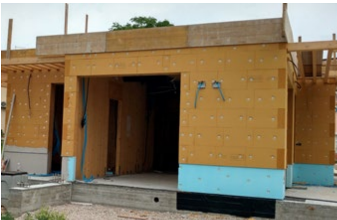
05-06 | Demonstrator building, Benevento. Construction phases: assembly of X-Lam panels (Cross Laminated Timber) and stratification of the external walls. The choice of the Fibertherm Flex 180 panel contributes to ensure a good thermal inertia thanks to its mass, making it suitable for the reference climate context
