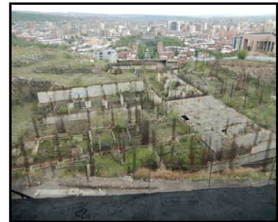
Top ruined areas over the complex staircase and under the Memorial terrace
