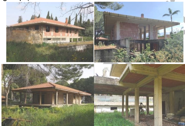
Fig. 04 Views of the unfinished buildings in the confiscated allotment (ph. A. Campagna, 2022).
